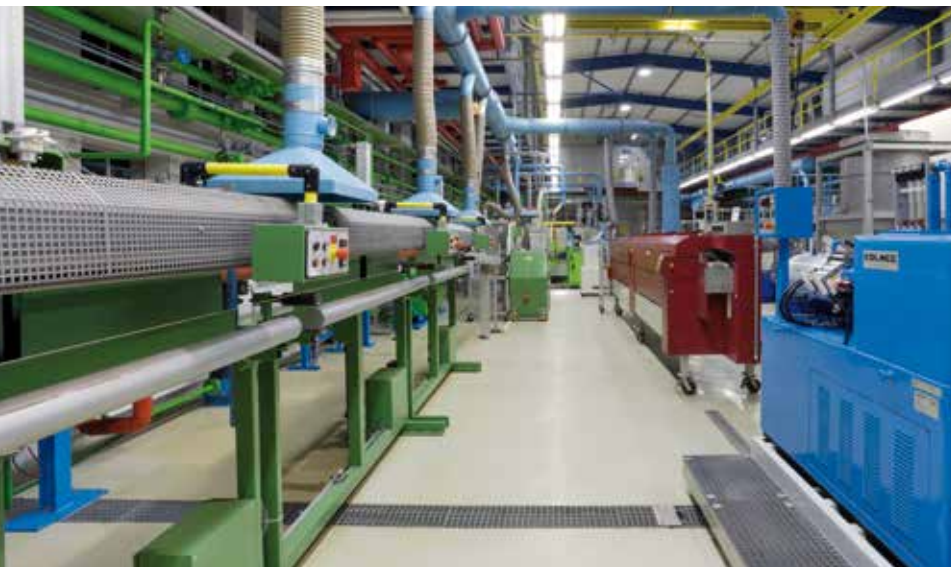
Cable production: extrusion with subsequent vulcanization in the infrared tunnel
