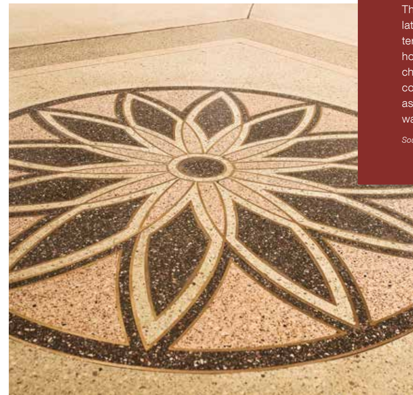
Impregnation does an especially nice job of bringing out the patina of the 140-year-old terrazzo flooring.
