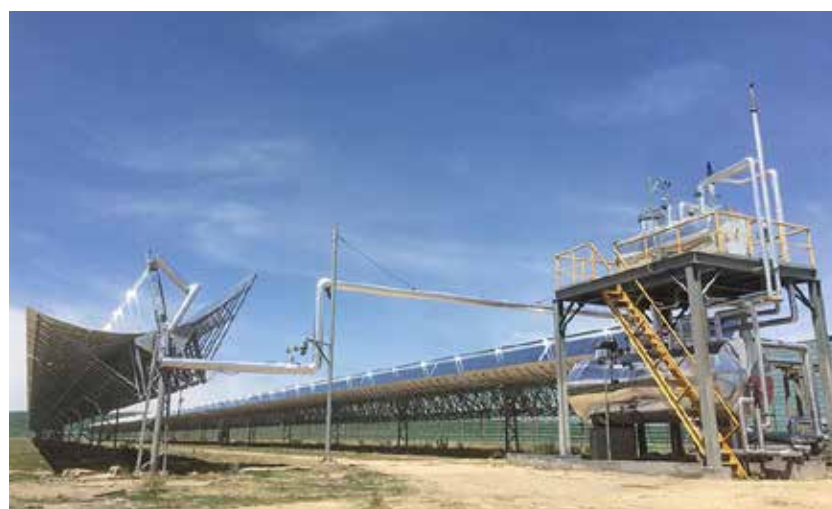
CSP (concentrated solar power) plants capture sunlight in parabolic trough collectors and use it to heat the heat-transfer medium flowing through a vacuum pipe.
