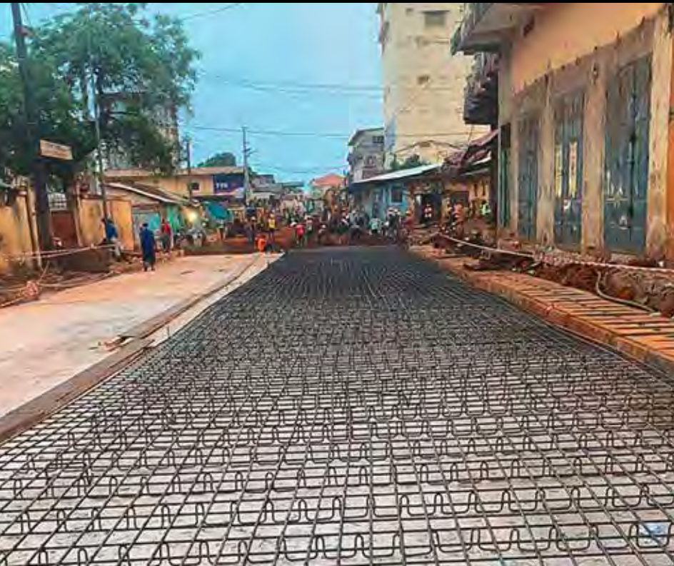
The concrete surface course is reinforced with steel – this is a complex solution that speaks to the high quality of the road structure.
