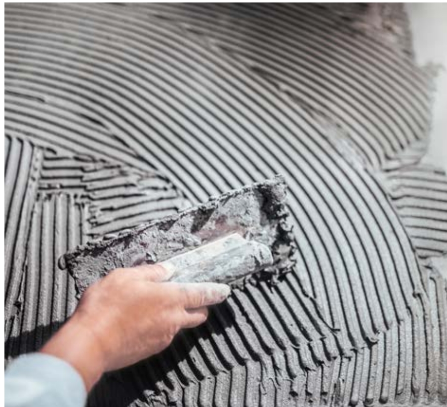
Before large-format tiles are installed, the walls or floor need very careful preparation and must be level.
