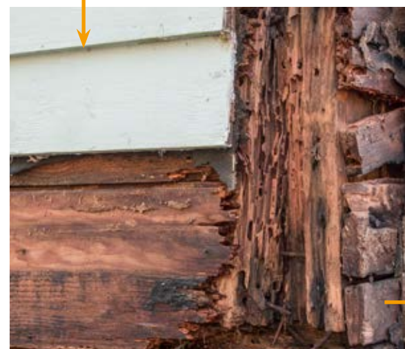
Top: Damage from ants to cracks in the walls of a house Bottom: Termite and rot damage to the foundation of a wooden house
