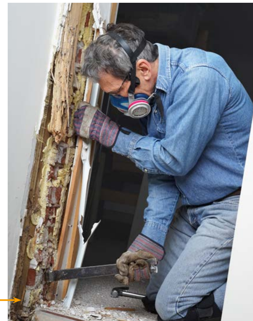
Exterminator removing damage caused by termite infestation in a house
