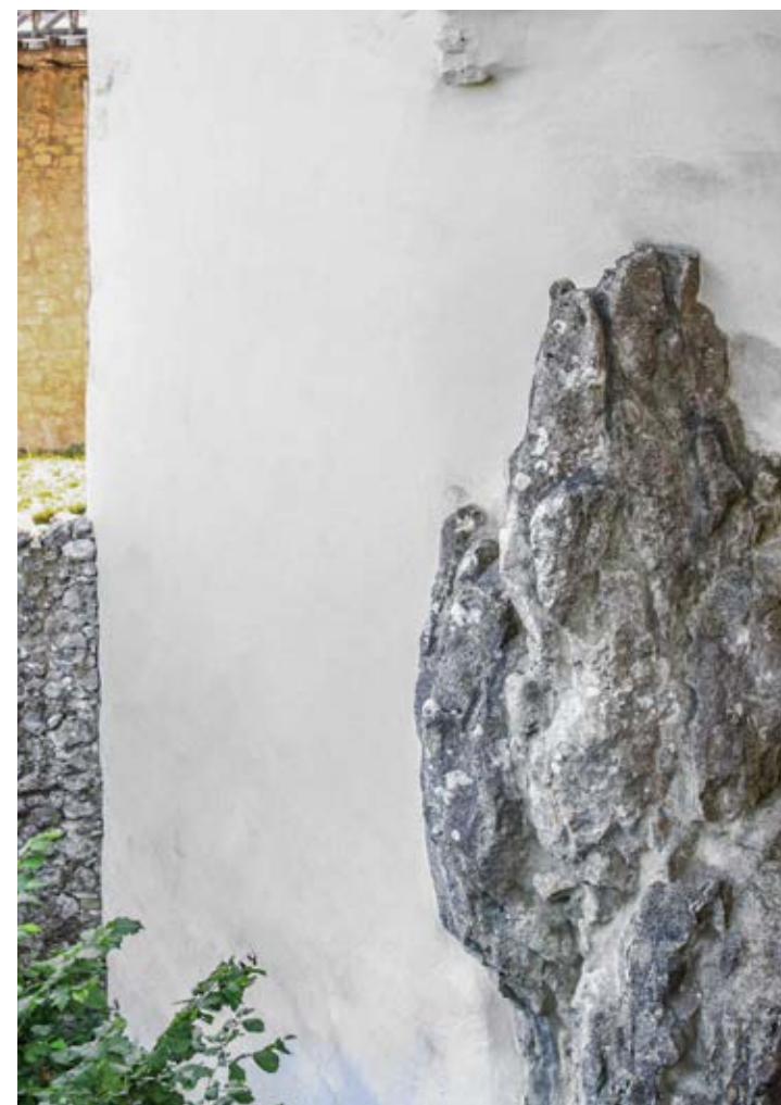
The rock beneath the stair turret of Prunn Castle now withstands all weathering influences.
