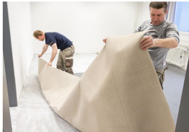
WACKER, too, has chosen a carpet from the Powerbacking line. It was installed in a meeting room at the Burghausen site.
