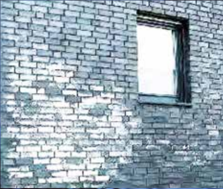
Water may cause efflorescence and salt damage due to hydration and crystallization.
