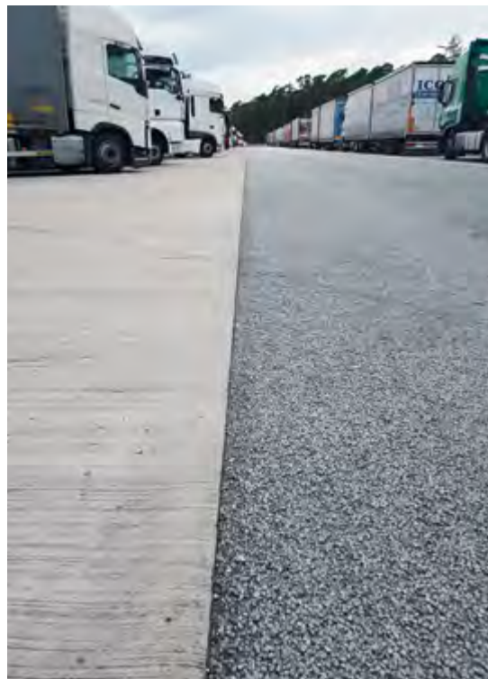
After two years of weather influences and maneuvering from trucks the concrete layer is still in excellent condition.
