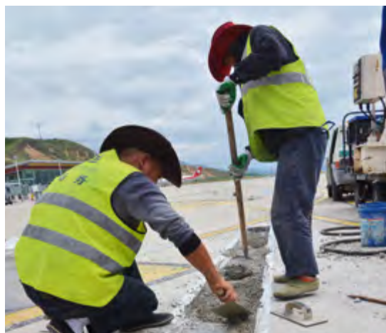
After: The use of modified concrete made it possible to repair the surfaces and have them ready for use again in just a few hours.
