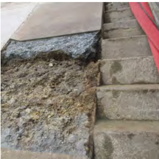
Before: Large-scale spalling made the canal in urgent need of renovation.
