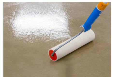
Coatings based on SILRES® BS 6920 are easily applied by wiping or rolling.
