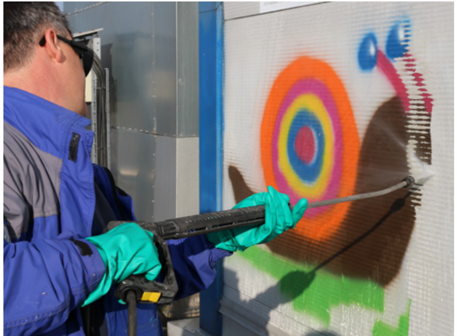
Removal of graffiti: Larger graffiti can also be easily removed using a high pressure cleaner with cold water.
