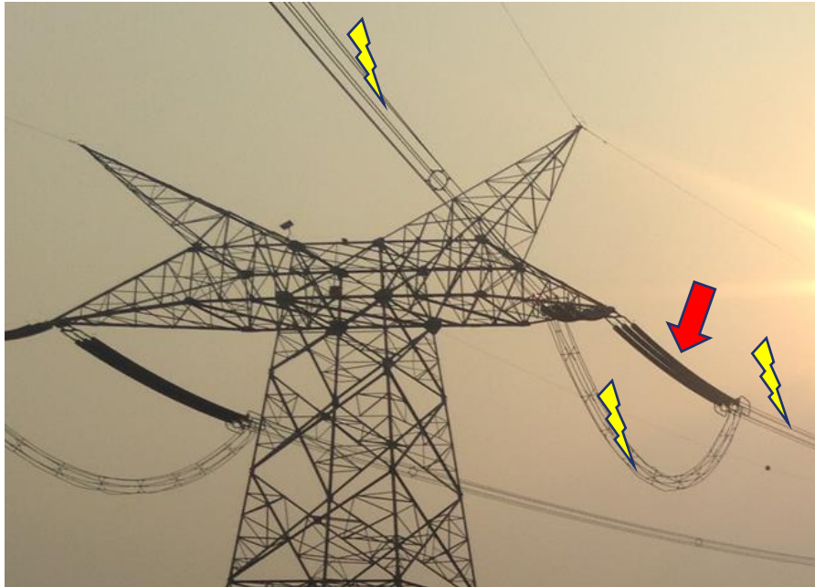
800 kV HVDC line – ceramic insulators
