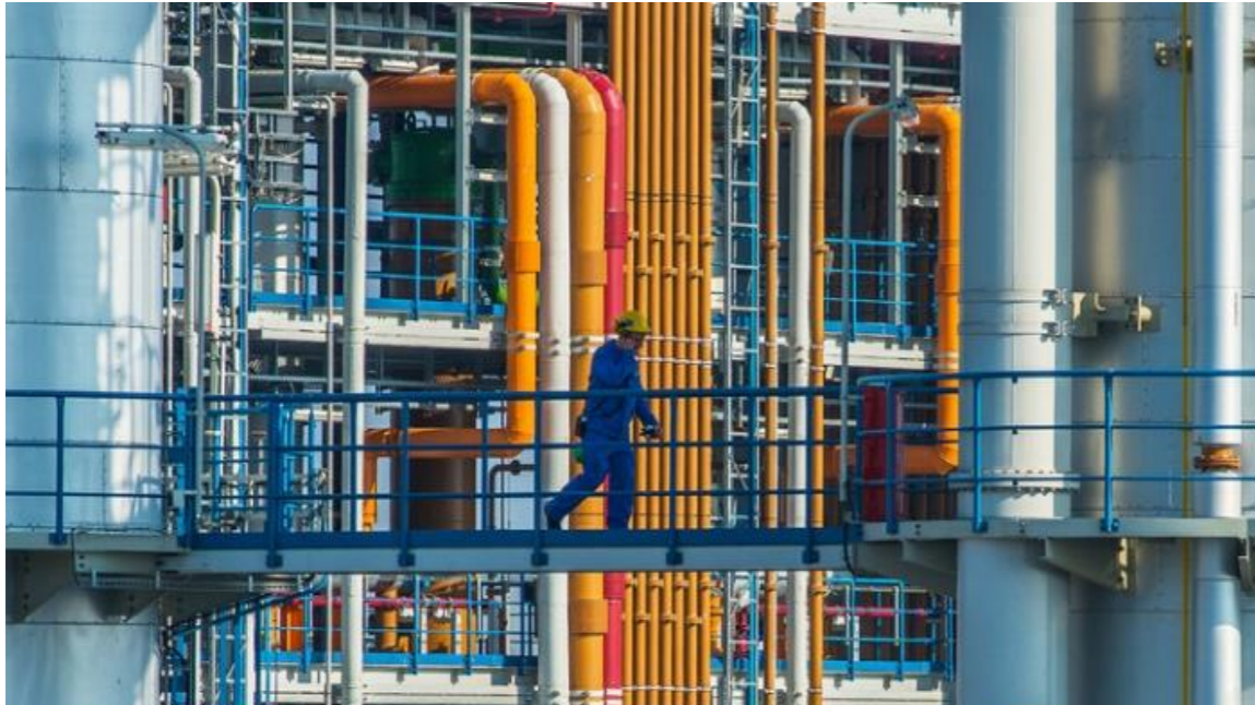
Section of polysilicon production plant in Nünchritz (Germany)
