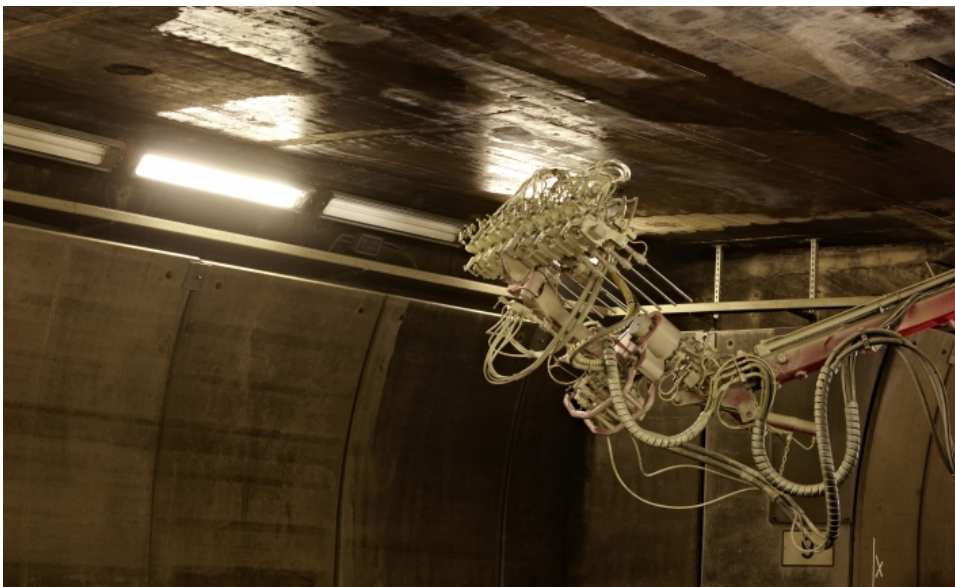
Renovating the Gotthard tunnel: specialists used compressed air to apply the silane impregnating agent. (Photo: Wacker Chemie AG)
