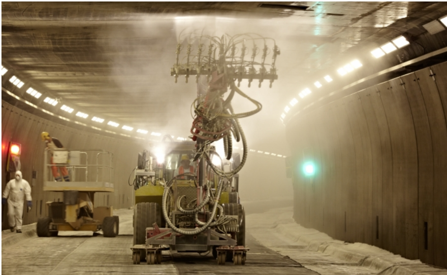
Completely closed to traffic: to provide protection against moisture and salt ingress, the ceiling of the Gotthard tunnel was impregnated in late September with a specialty silane cream made by WACKER, the Munich-based chemical group. (Photo: Wacker Chemie AG)
