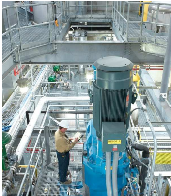
Dispersion reactor in Calvert City (USA)
