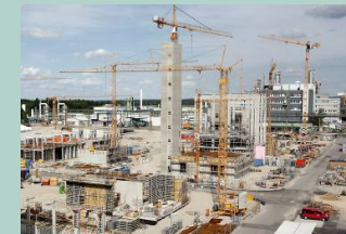
June 2007 New gas recycling systems
