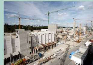
June 2007 New reactor hall
