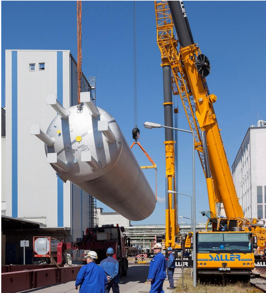
30-meter-high dispersion storage silos with a capacity of 330 cubic meters each
