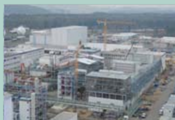
December 2008 New reactor hall
