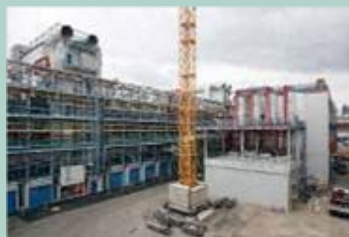
July 2009 Deposition reactor hall
