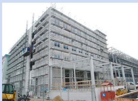
Polysilicon expansion in Burghausen
