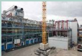
July 2009 Deposition reactor hall
