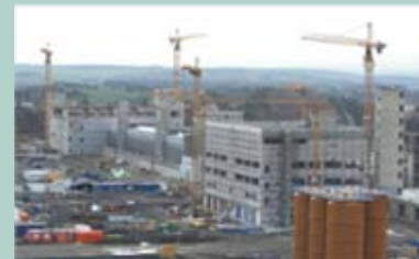
November 2009 Deposition reactor hall
