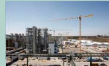
April 2008 New distillation system
