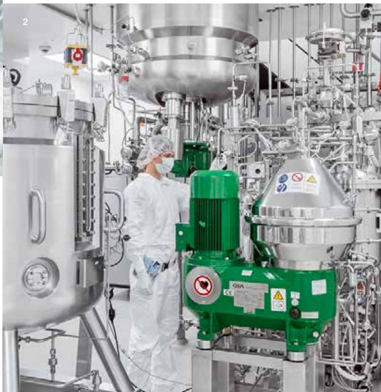
2 Bioreactor in Wacker Biotech's clean- room: Actives for pharmaceuticals are produced here in extremely pure form.
