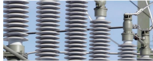
Insulators and cables
